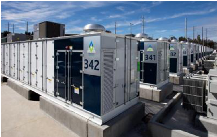
Figure 7: San Diego Gas & Electric's 30 Megawatt Escondido Energy Storage Facility
